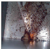
Sludge in tank
